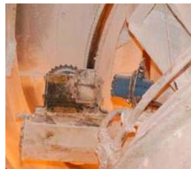
Four 648 (single point) Smart Wireless Temperature Transmitters were placed inside the silos to measure bearing temperatures and motor currents.
