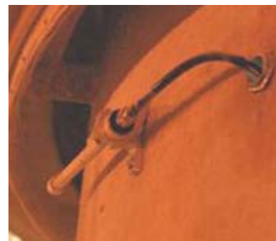
A remote antenna on the center rotating shaft inside the sugar silo allows the wireless instruments to communicate with the Smart Wireless Gateway located outside each silo.
