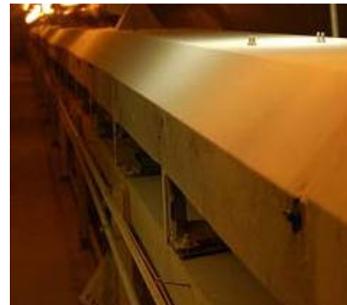
Each of the nine conveyor belts had four bearing temperature measurements and four rub block temperature measurements that were handled by one 848T FOUNDATION™ Fieldbus High Density Temperature Transmitter.
