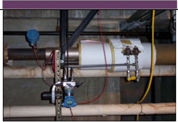
Figure 2. 1495 Orifice Plate (check meter) installed downstream of the 3095MFC Compact Orifice Mass Flowmeter
