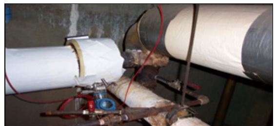
Figure 1. 3095MFC Conditioning Orifice Mass Flowmeter installed two pipe diameters after two out-of-plane 90 deg elbows.
