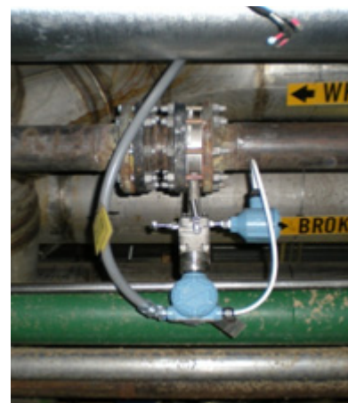
Figure 2: No new piping modifications or welding was required in this quick installation.
