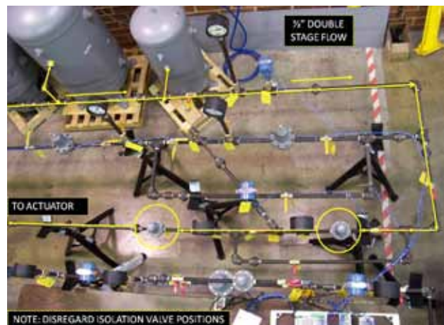
Figure 4. Close-up showing flow from reservoirs through 1/2" double stage flow circuit
