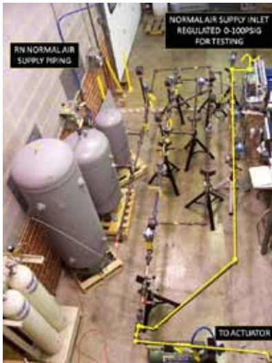
Figure 2. Overall test set up highlighting the normal air supply circuit
