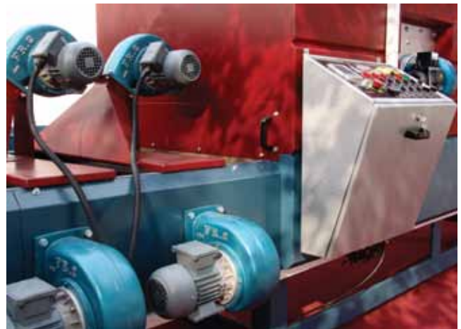
Aside from compressors and turbines, condition-based maintenance technology can also be applied to other essential production assets such as motors, fans and pumps.
