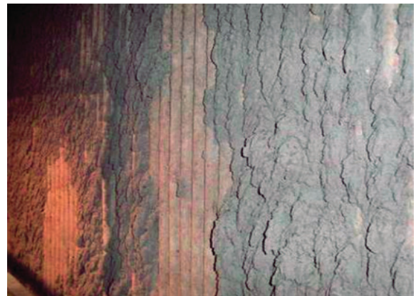
Figure 6 - Slag formation on boiler tubes.
