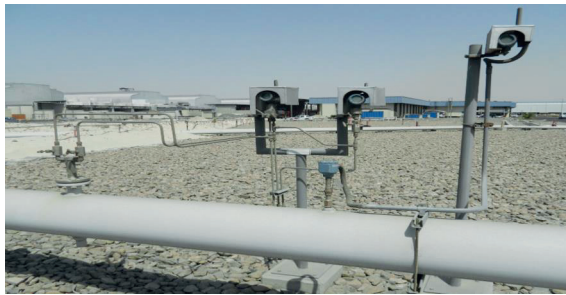
Fig 4. EGA Dubai wireless sensors for digital transformation energy efficiency
