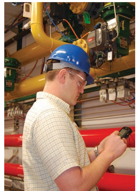
FIG. 2. A technician can run valve diagnostic tests using a handheld device, a laptop or from the control room.
