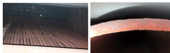
FIGURE 2: Damage caused by poor performing attemperators can include warped tubes (left) and cracked attemperator liners (right) due to quenching.
