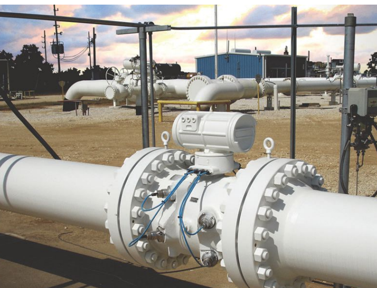
Figure 4: This photo shows an ultrasonic meter installed in a natural gas field. Courtesy: Emerson Process Management
