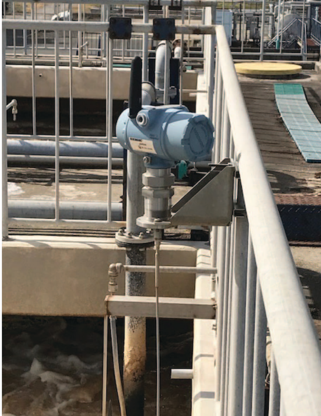
The Rosemount™ 3308 Wireless Guided Wave Radar installed over the concrete pit
