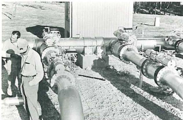
Robotarm Actuators used as ball valve regulators in a gas storage field.
