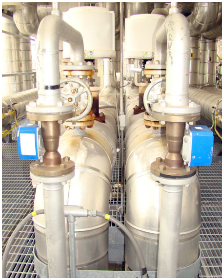
BEFORE: Rotameter Installation
