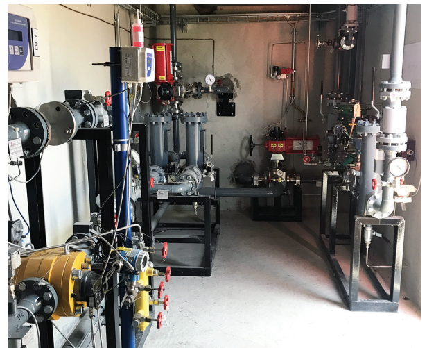
REMI Station internal view
