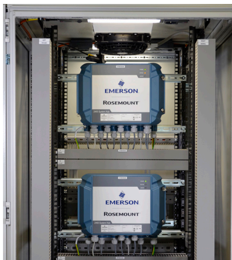
System hubs are often installed in Emerson supplied ready-made tank gauging cabinets.
