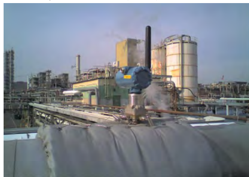
Figure 10.15: Direct mounted Rosemount 3051SFC wireless flow meter on an exterior steam application where the steam temperature is 365 °F (186 °C).
