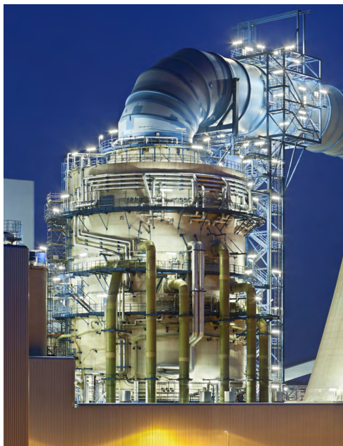
Figure 4.10: A utility scrubber for emissions reduction.
