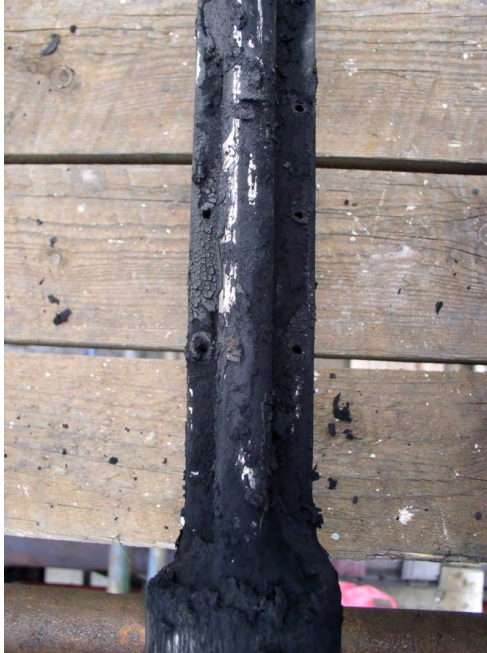
Figure 10.44: Close up of the solids buildup on the base of the Stack Annubar sensor exterior. Required maintenance is needed to clean the sensor periodically.
