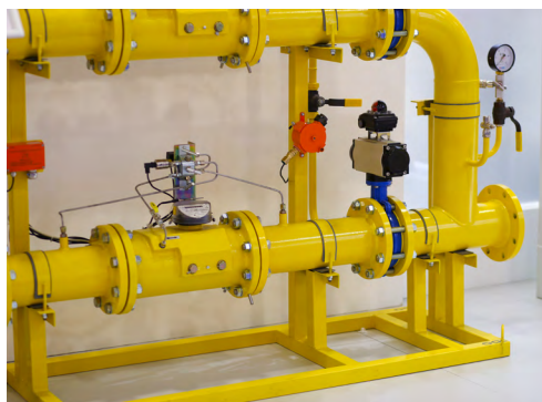
Figure 4.12: A furnace fuel control skid.
