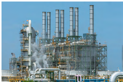
Figure 5.7: Refineries have many flow meter applications that typically require stringent design and qualification testing.
