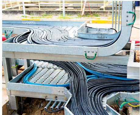
Figure 10.17: Conduit and cable tray.
