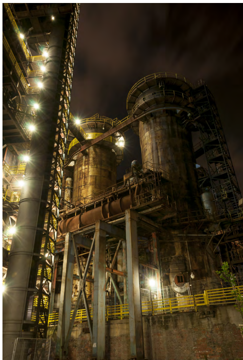
Figure 5.3: A blast furnace, where cooling systems should be monitored for proper flow to prevent damage or hazardous conditions.
