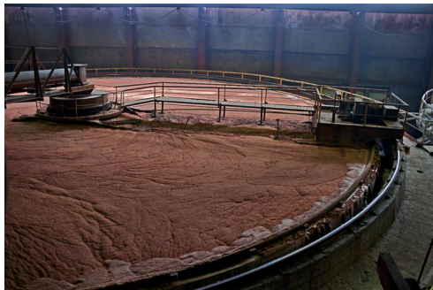
Figure 4.14: A dissolved air flotation cell for separation of metals.
