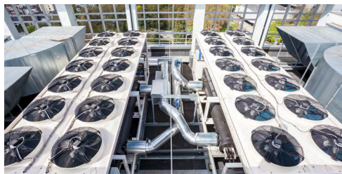
Figure 4.9: An air-cooled chiller for an air conditioning system.
