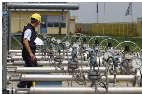
Figure 5.9: A midstream flow metering and regulation station.
