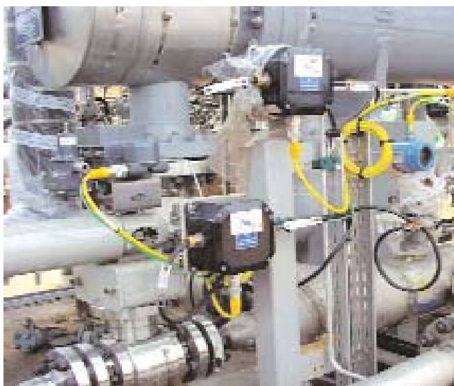
Fig. 4. On the Malampaya platform's IS installations, the additional expense of quick-disconnect cables was offset by speedier installation and shorter transmitter replacement times.
