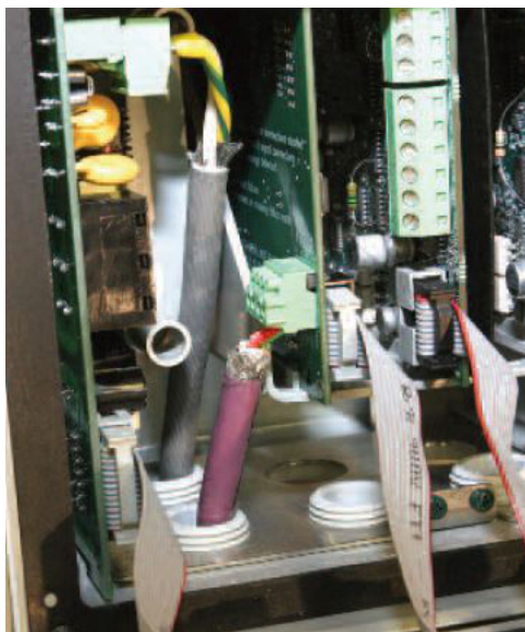
Figure 12-5: Complete PROFIBUS Board Installation with Ribbon Cable Attached
