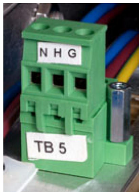
Figure 5-8: AC/DC Termination Block
