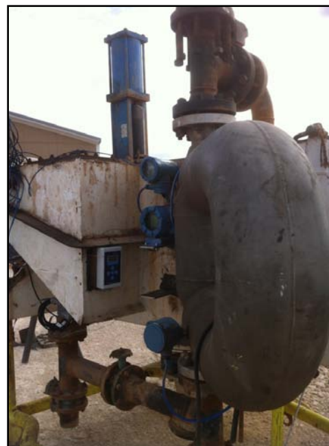
Figure 10. Example of a Coriolis installation in a flag position for RCD rig type
