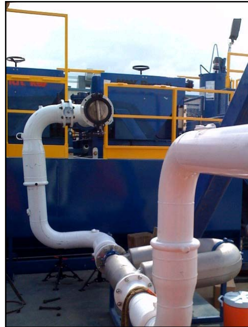
Figure 9. Example of a Coriolis installation at a 5 degree incline for RCD rig type
