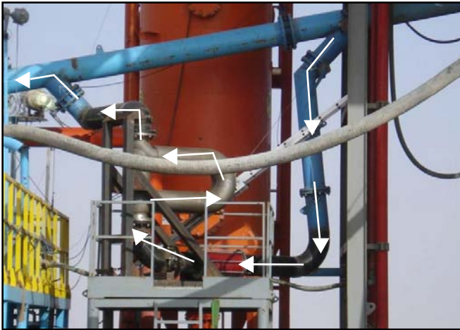
Figure 11. Example of a Coriolis installation for a conventional (bell nipple) rig type. Note the bypass and flow direction through the Coriolis from bottom to top.
