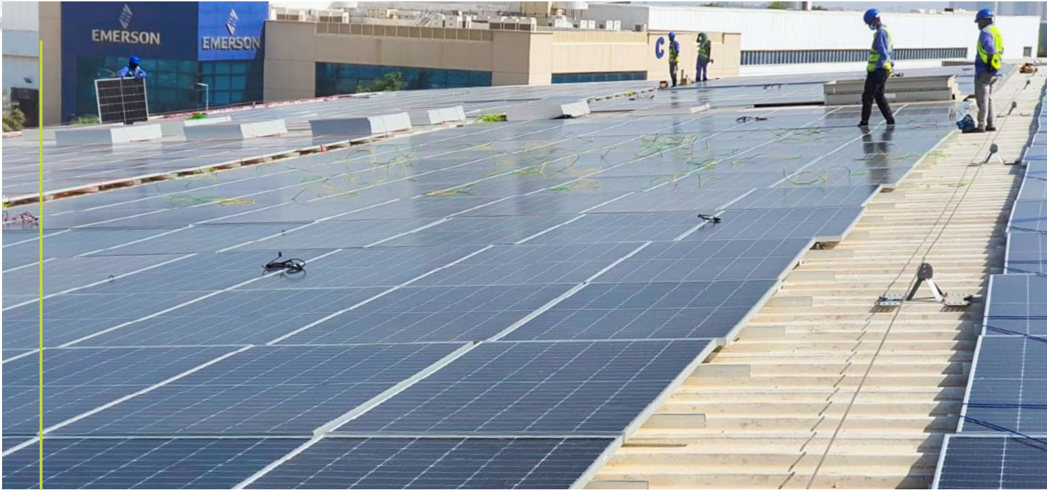
Emerson Dubai campus recently installed an on-site solar system that provides over half of its daily electricity usage.
