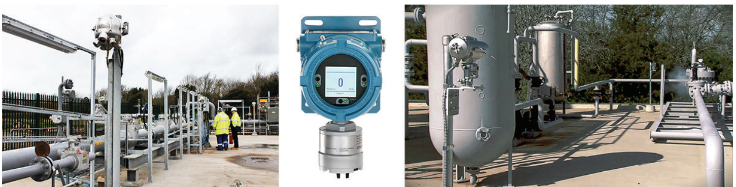
FIG. 8. Gas detectors use different approaches, including (left to right): acoustic, point and open path.
