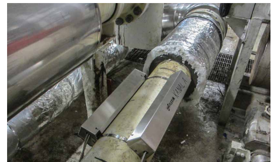
The final gas flow measuring point with the transducers installed in the Variofix C transducer mounting device.
