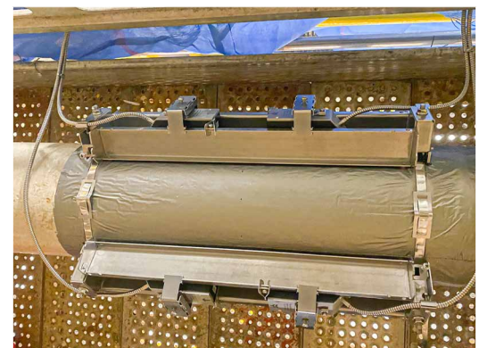
The measuring point with two pairs of clamp-on ultrasonic transducers type GSK during installation
