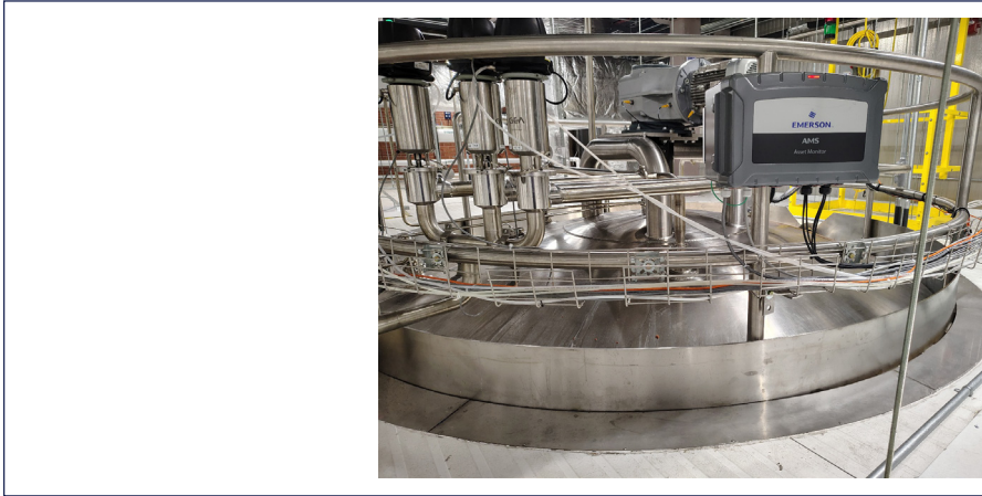
Figure 4: This 10,000-gallon tank is part of the plant's aseptic line and uses an agitator turned by means of the motor and right-angle gearbox visible in the photo. The AMS Asset Monitor is also visible along with three of its four connected sensors on the gearbox and inboard end of motor.
